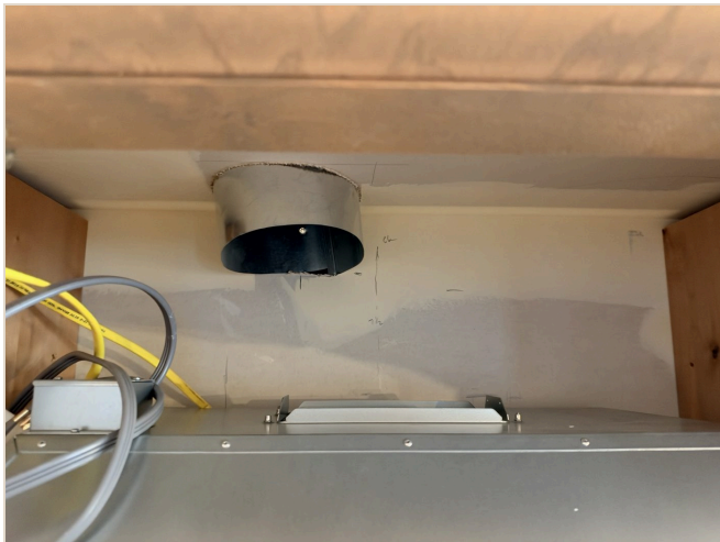
PHOTO 1 Existing 8" duct stub hanging below the ceiling, top of hood below
